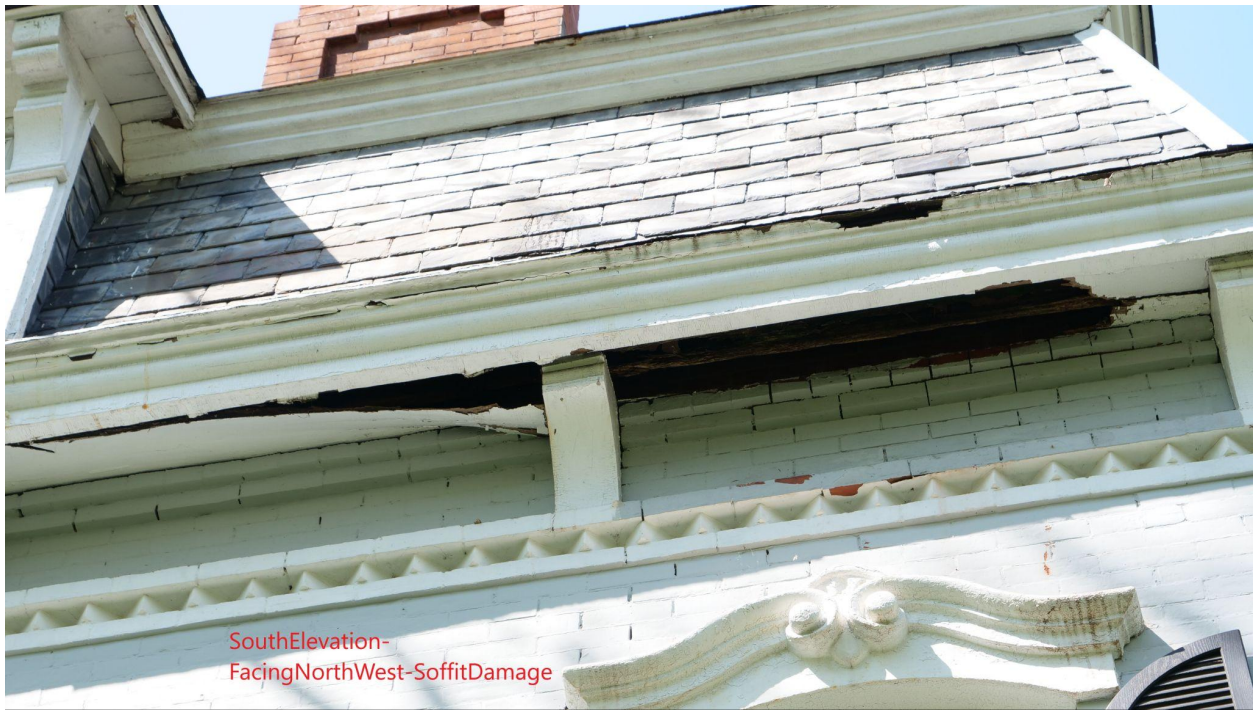
SouthElevation- FacingNorthWest- SoffitDamage-2
