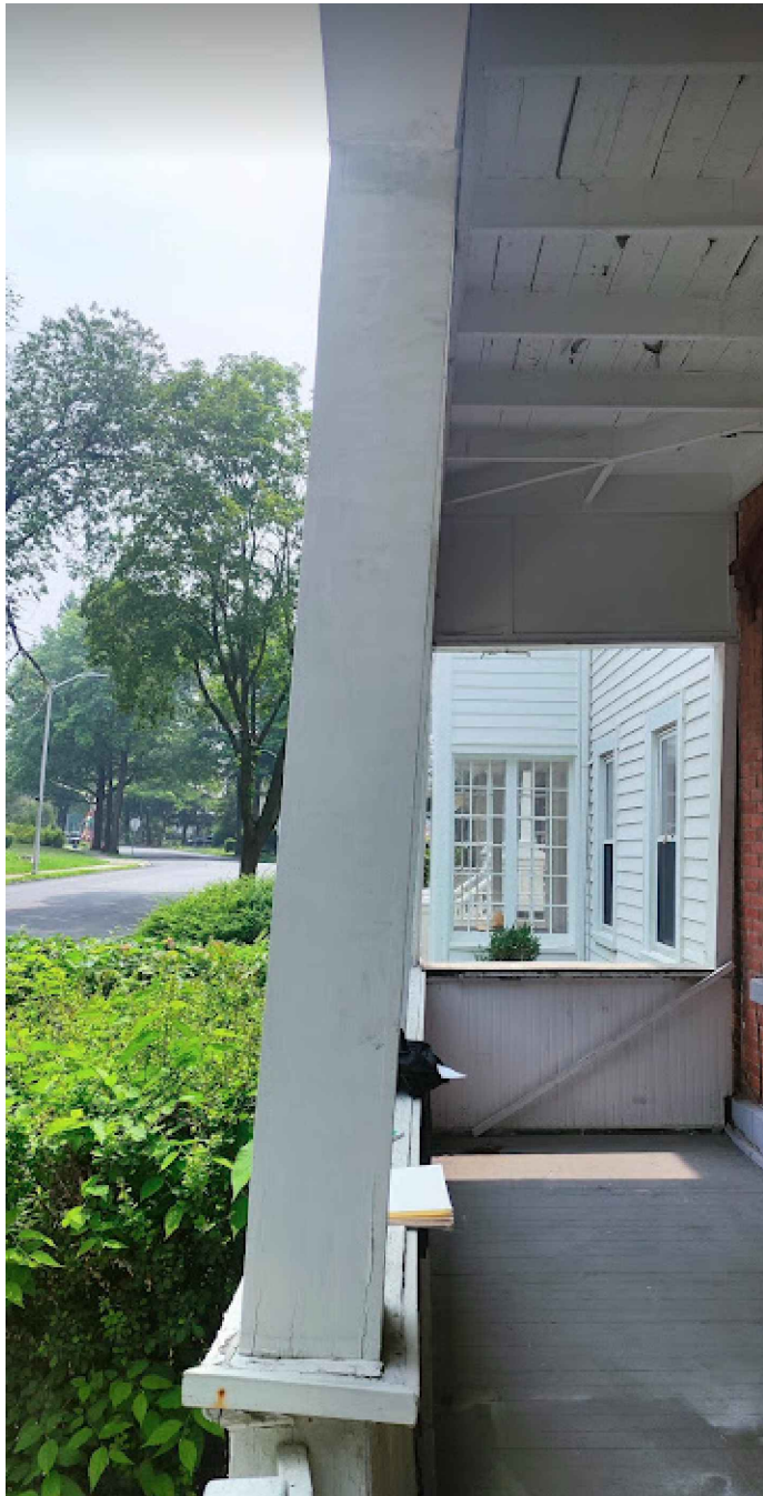
EXISTING COLUMN BUCKLING
