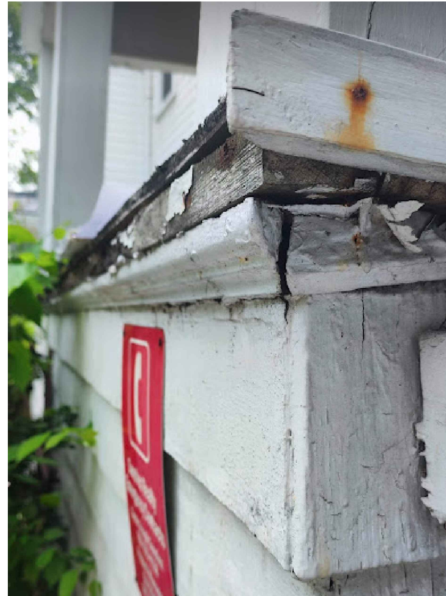
EXISTING NON-HISTORIC HALF WALL WITH ROTTEN MOLDING
