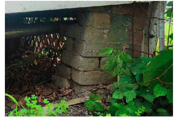
CRUMBLING BRICK PIERS
