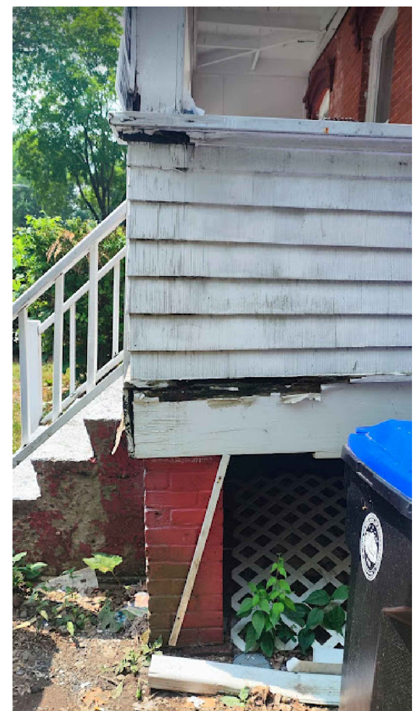
EXISTING NORTH ELEVATION ROTTED BOARDS/ SETTLEMENT
