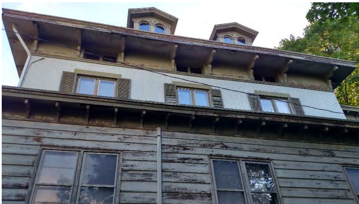
Photo 5: Upper stories on west elevation. The lower attic windows, cornice brackets and eaves have all been replaced with mid-20 th century materials.
