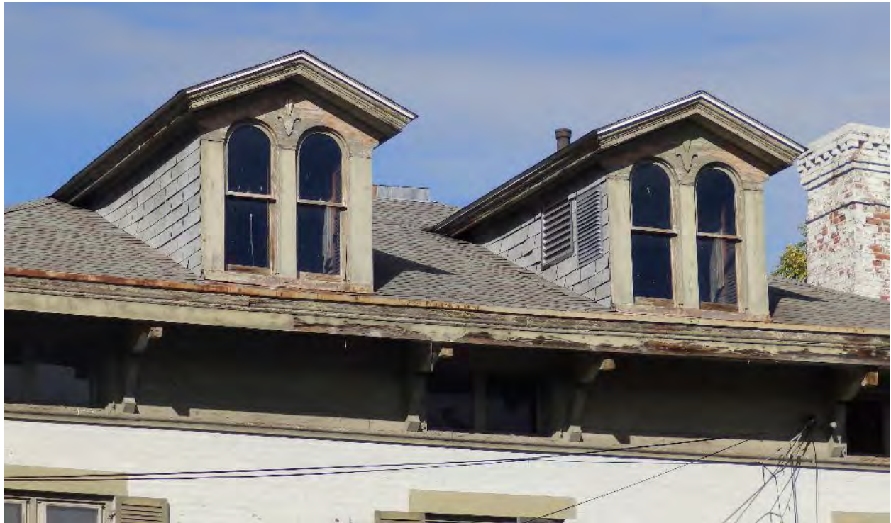
Photo 6: Arched dormers located on the east elevation. The dormers originally had single pane arched windows on the sides of the gabled dormers. These windows have been covered with asphalt shingle (see left gable) or replaced with air vents (right gable).
