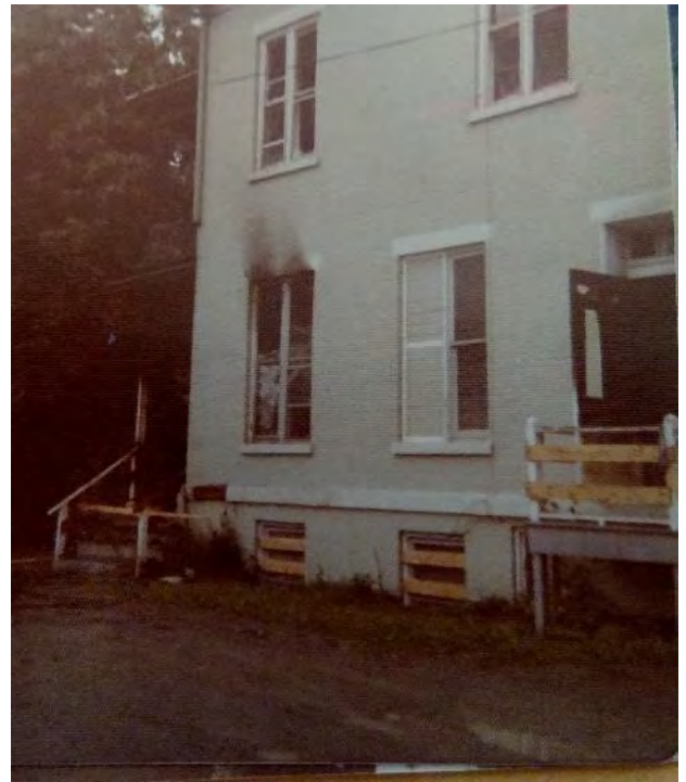
Photo 10: View of the eastern elevation after the 1979 fire. (Source: Poughkeepsie Day Nursery Files: Adriance Memorial Library).
