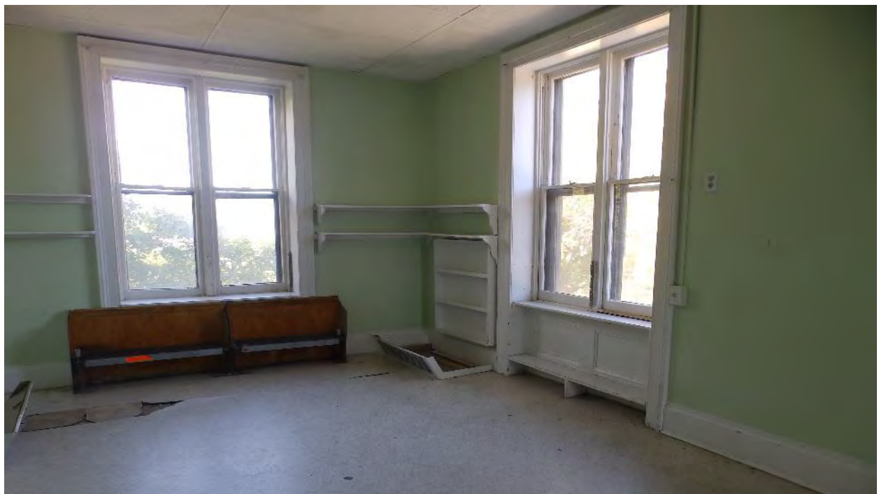
Photo 28: This room is identified on the Second Floor Plan as 202. Wooden trim patching in the baseboard suggests that a fireplace was once located in the wall in the right of the photo.
