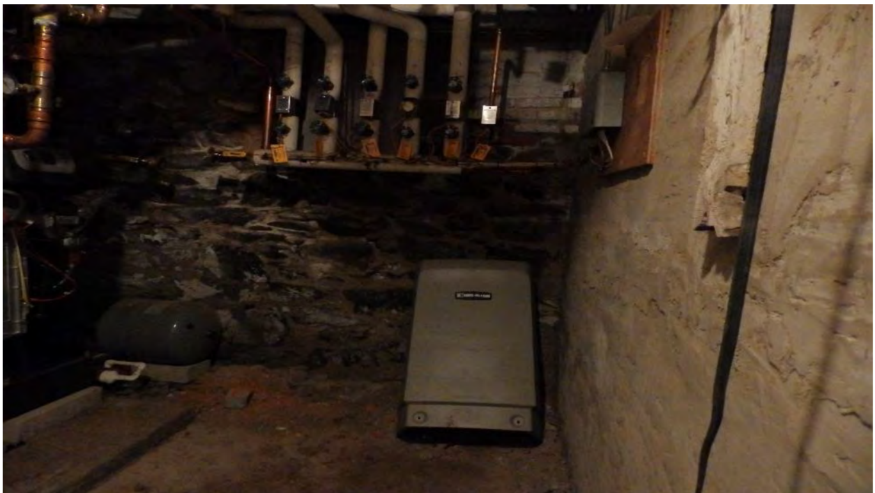
Photo 18: Room identified on floor plan as Mech 05. The heating system and furnace indicate that the structure has been extensively renovated to accommodate modern heating technology.
