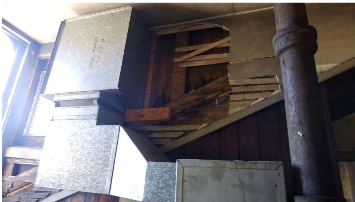
Photo 35: Cast iron pipes and aluminum duct work located in the attic illustrate the extent to which the heating systems within Hill House have changed during the 20th century.
