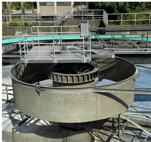
Figure 3-2 Energy Dispersion Well and Feedwell
