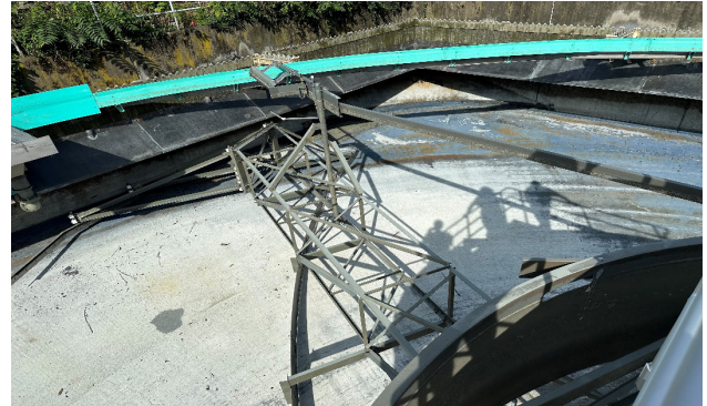
Modified secondary clarifier mechanism and relocated density current baffles.
