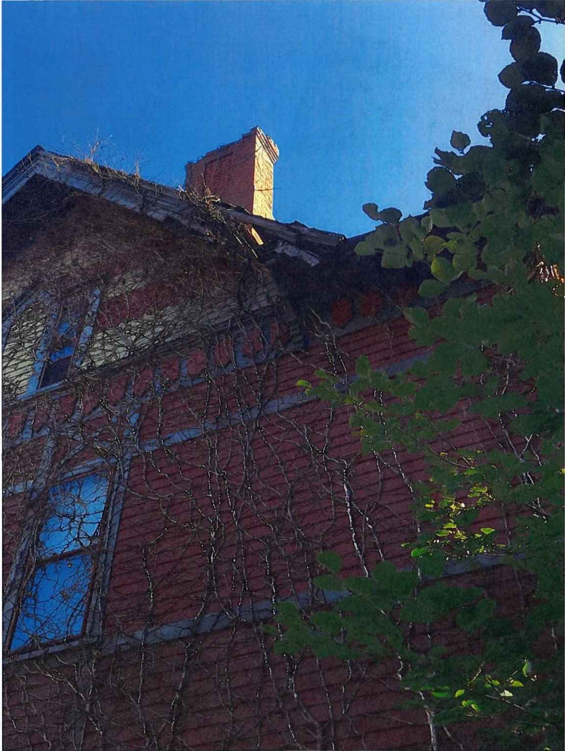
Detail: 130 Academy Street north wall , rear side yard view: pitched roof and chimney damage
