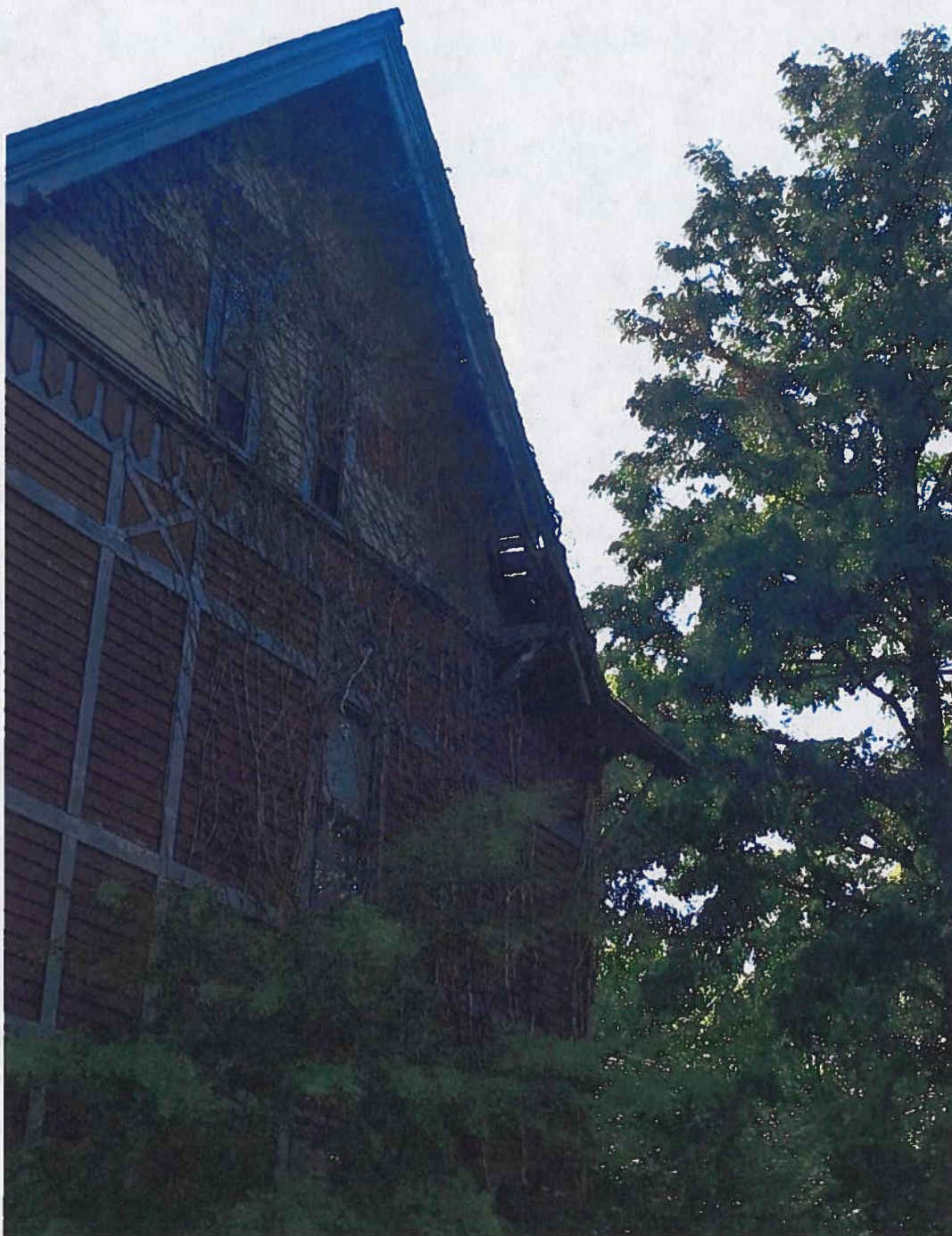
130 Academy's north wall , side yard view of rear pitched roof damage
