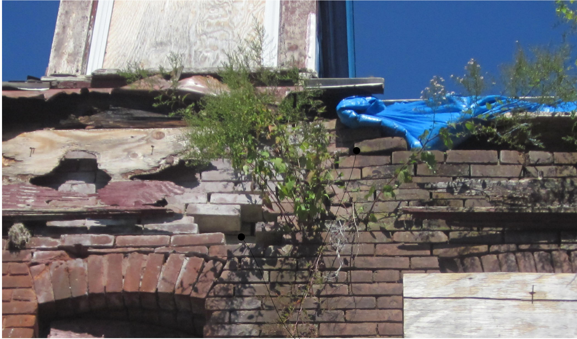
2 SOUTH FACADE - LOOSE & MISSING BRICKS N.T.S.
