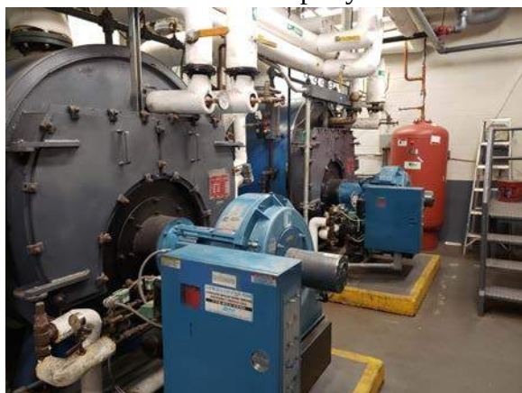
View of Heating Oil Fired Boilers
