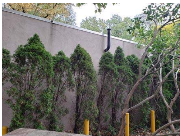
Heating Oil Storage Tank Building on North Side of Property
