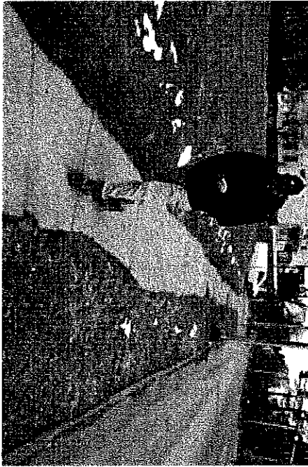
Broken sidewalk on Mansion Street, just north of Cottage Street
