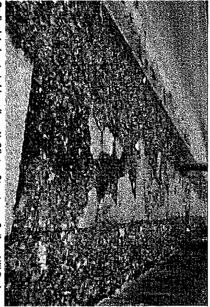
Badly deteriorated sidewalk on N. Clinton Street near College Hill Park
