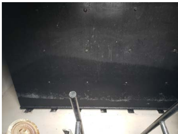
Fuel Tank, Tank House Floor, and Fill Port
