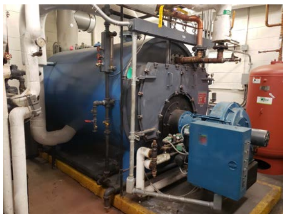
Heating Oil Fired Boiler
