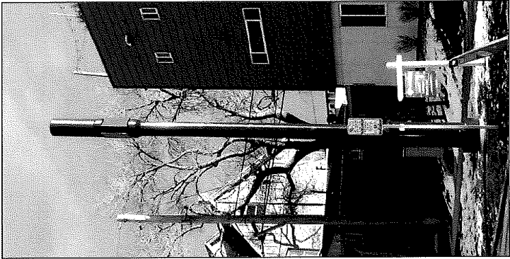
4G + 5G Small Cell in a Concealment Pole
